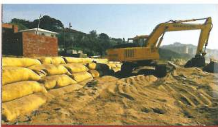
Placement of GSC bags on the beach as part of a GSC revetment structure in KwaZulu-Natal
