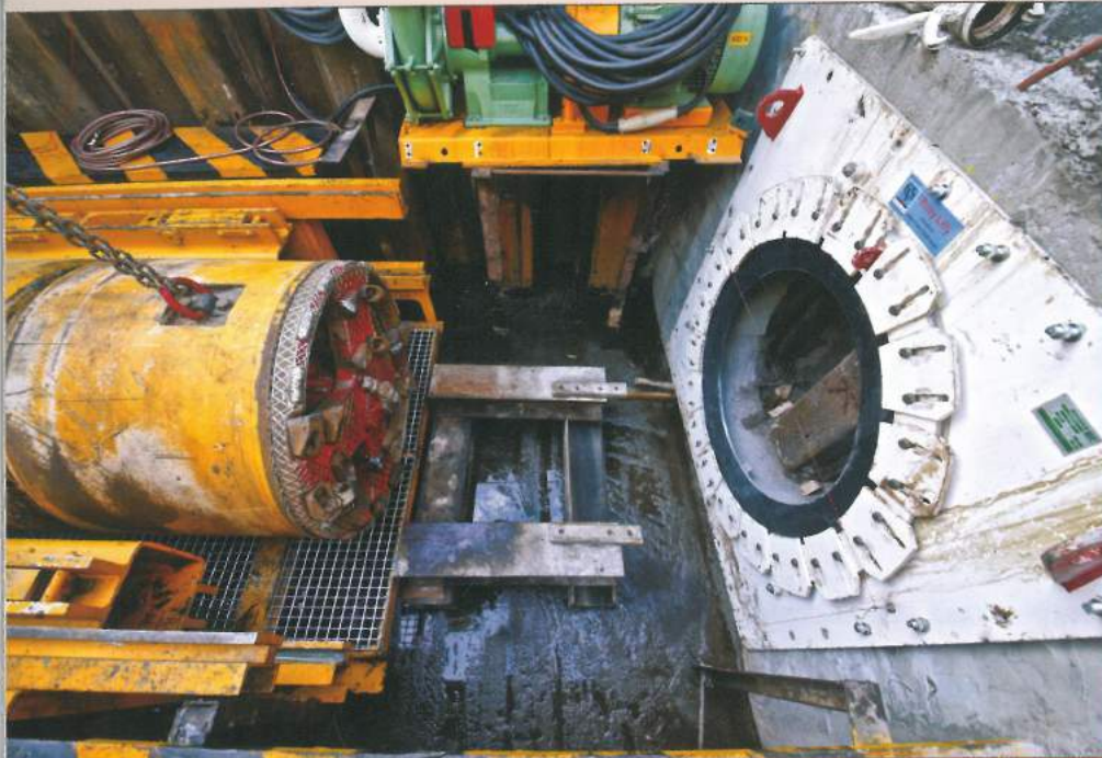
A TBM was used to mechanically cut and remove soil from the jacking face by means of a rotating cutting head and pumped slurry conveyance system
