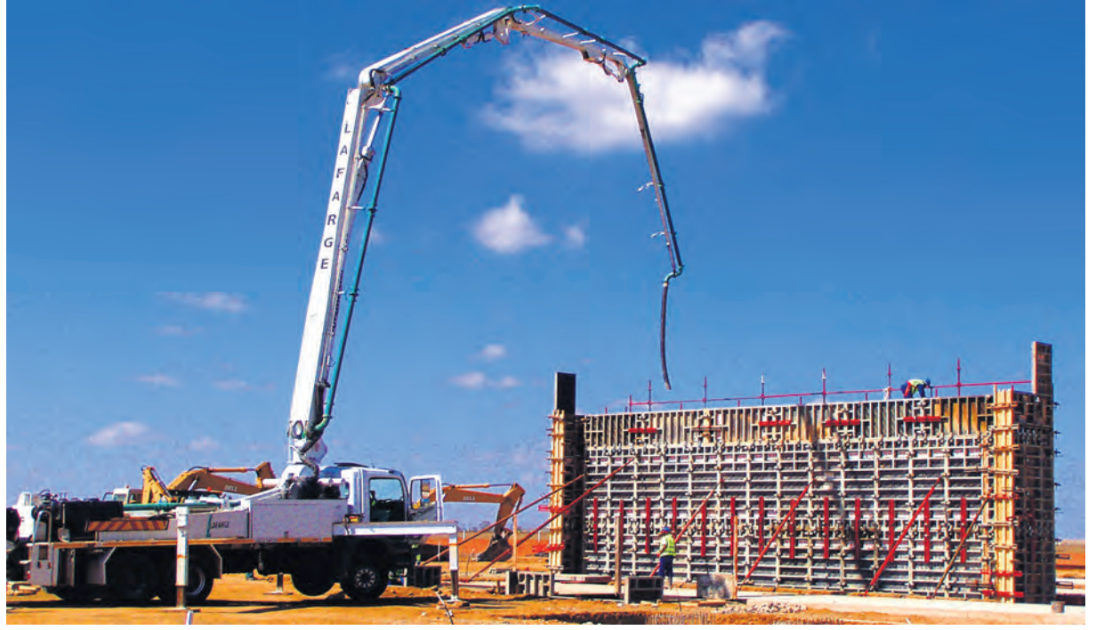
The construction of the 765 kV Perseus blast wall in Bloemfontein is part of CSV's commitment to building a greener SA.
