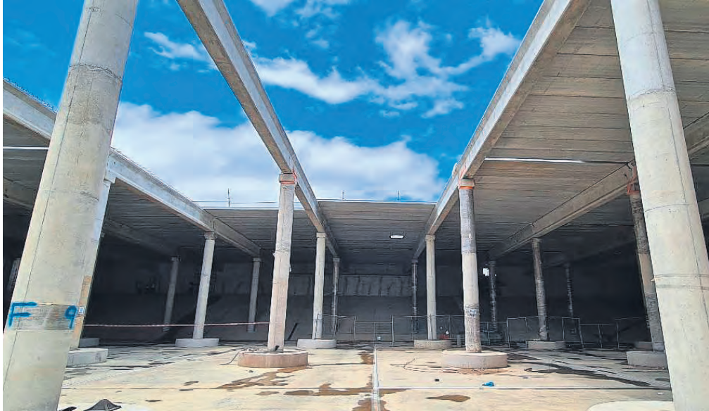
During the works at the Contermanskloof Reservoir, molding sloping slabs proved to be a challenging and time-intensive task.
