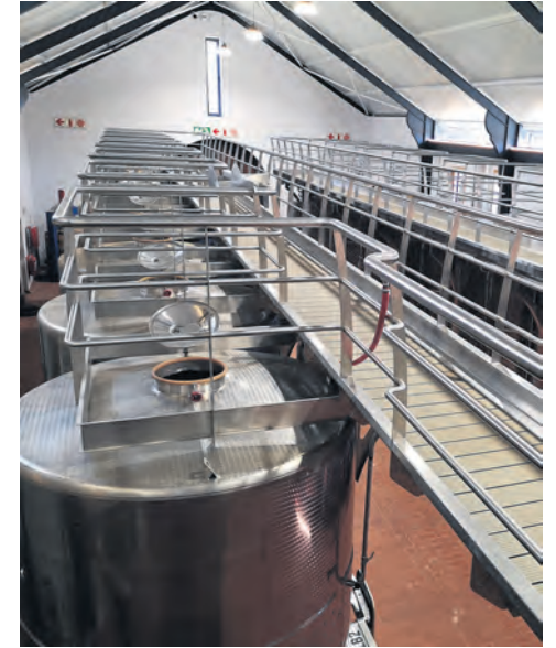
CSV had to modify an existing farm store to tie it into the barrel maturation area, which served as the fermentation area.
