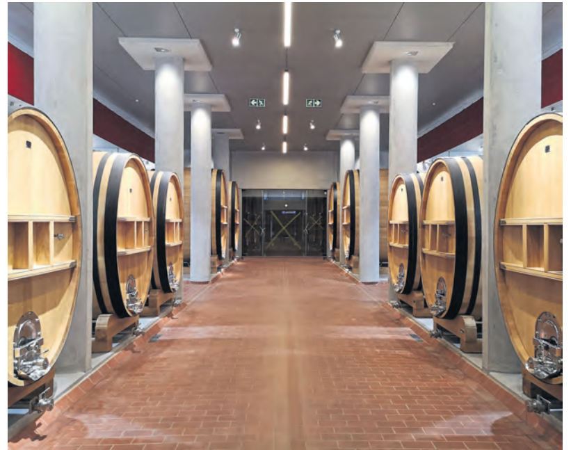
Forty oval-shaped precast columns with bases needed to be installed in the barrel maturation area at Cordoba.
