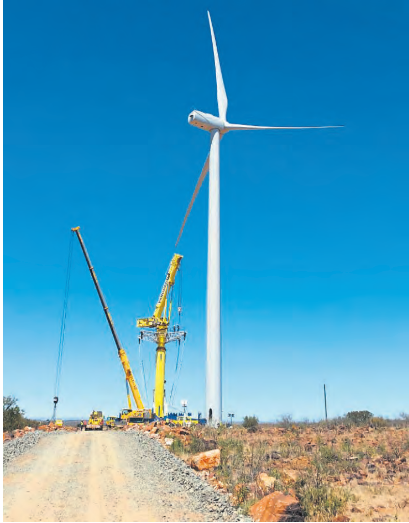
The Longyuan Mulilo De Aar 1-2015 1 MW Turbine project.
