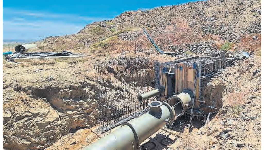
The incoming pipeline at the reservoir was constructed, in total, using 19 m sections welded together to create the 1 000 mm diameter steel pipe.
