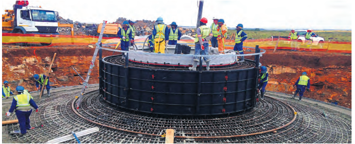
CSV was tasked with constructing a concrete base for wind farm turbines at the Longyuan Mulilo De Aar 1 project.
